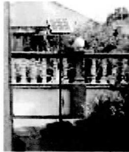
Solar Collector Panel
