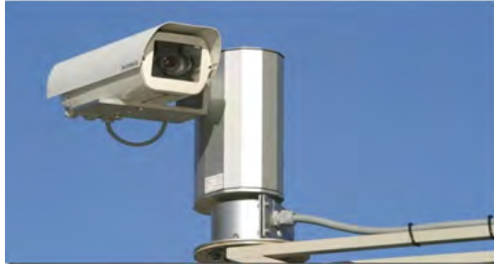
Figure 9: Red light enforcement camera
