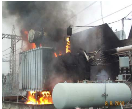
Figure 1.1 Damage to the transformer at TNB substation
