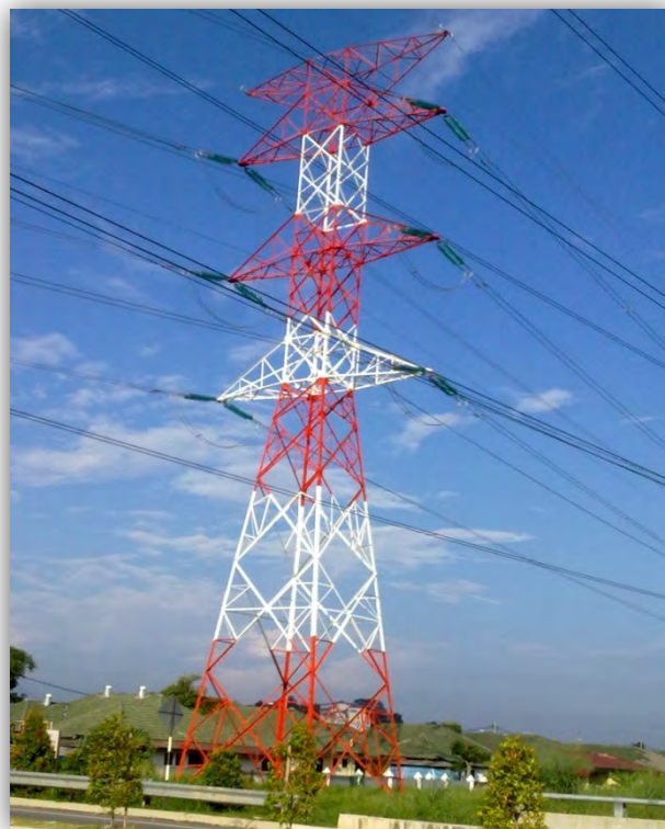
Figure 2.2: Example 275 kV double circuit transmission line
