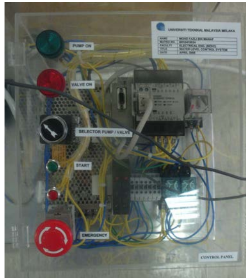
Rajah 5.6: Panel kawalan
