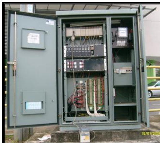
Figure 2.7: Completed controller wiring (Samsudin, 2007)
