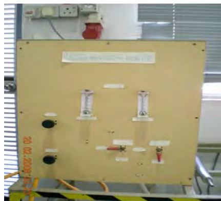
Figure 3.19 Control meter of gas flow rate
