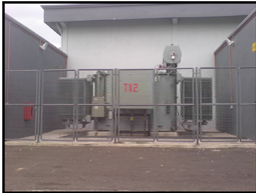
Figure 1.2: Power transformer 30 MVA (33/11 KV) in operation.
