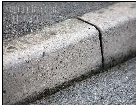
Figure 1.1: Road side curb before painting ( Majlis Perbandaran hang Tuah Jaya)
