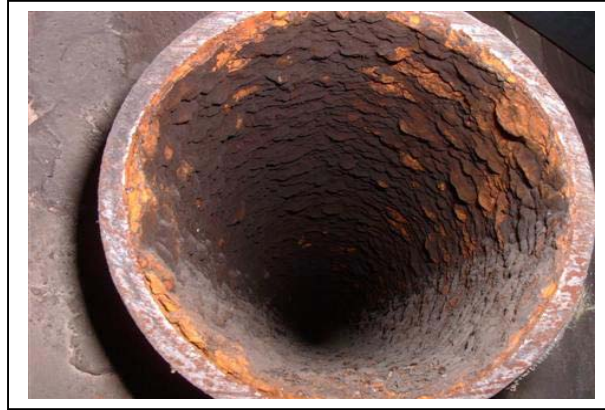
Figure 1.0: Internal Corrosion on Pipeline (Source: http://www.corrview.com/service_03.htm )
