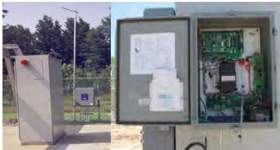
Figure 2.1 : Remote terminal unit in distribution panel box
