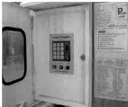
Figure 1.6: Control room for Paternoster System.
