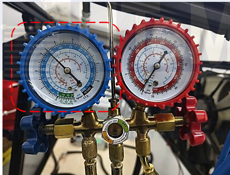
Figure 4.3 System pressure test indicator (Day 1)
