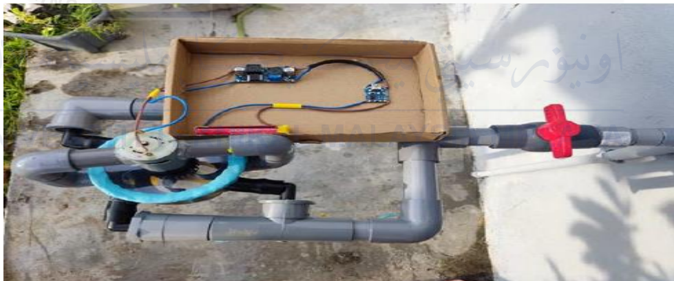
Figure 2.13 Pico hydro connected in domestic area
