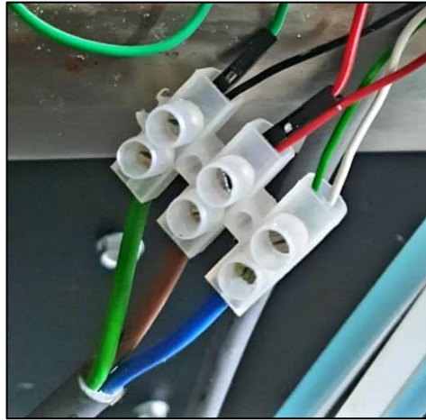
Figure 4.4: Wires from the laundry machine.
