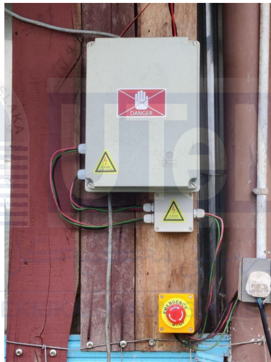
Figure 4.12: Power Distribution Box
