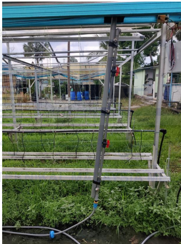
Figure 4.42: Pesticide Spraying Pipe Deviation Problem
