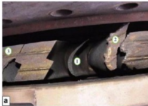
Figure 1.1: Upper Views of the Failed Blade and Surrounding (Source: Poursaeidi, E. et. al. (2007))
