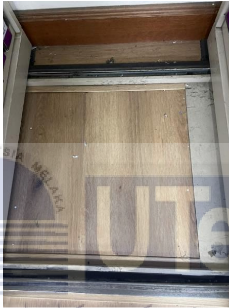
Figure 4.2: Unclean floor in file storage area
