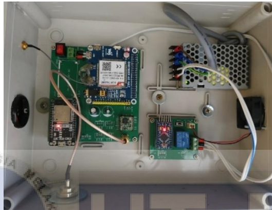
Figure 4.12: Gateway Node Casing
