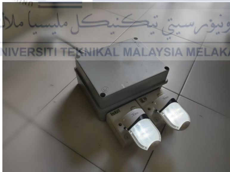
Figure 4.4.4 Both Power are turn On
