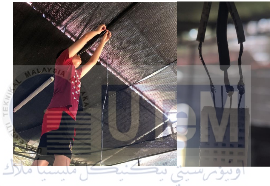
Figure 4.17 Installation DHT22 on ceiling mushroom house.
