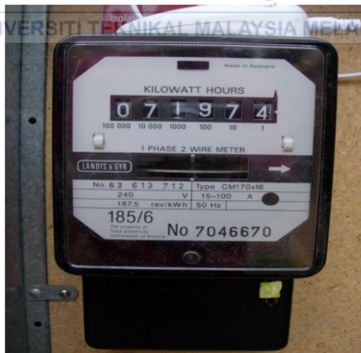
Figure 2.1 Traditional Electrical Meter [6]
