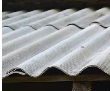
Figure 2.6: Asbestos cement sheets (Edwin Raczko et al ., 2022)
