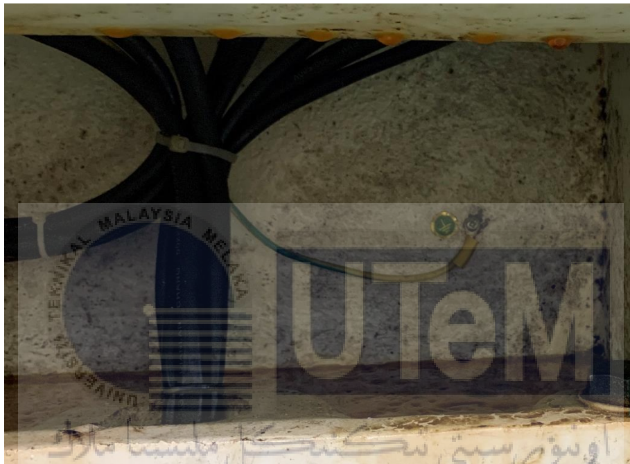
Figure 2.25 Example of lubrication issues
