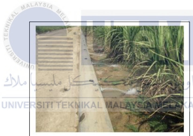
Figure 2.2 Hydro-flume with Adjustable out-let valves for Furrow Irrigation[9].
