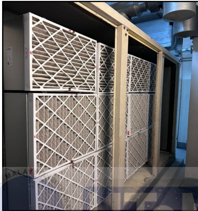
Figure 4. 7 Filter in AHU
