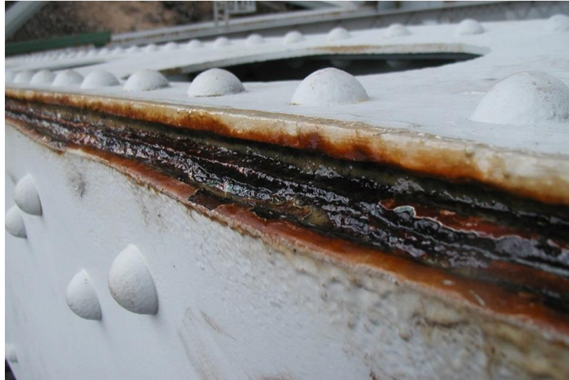
Figure 2.10 Crevice corrosion that occurs (Steel Fabrication Services, 2021).
