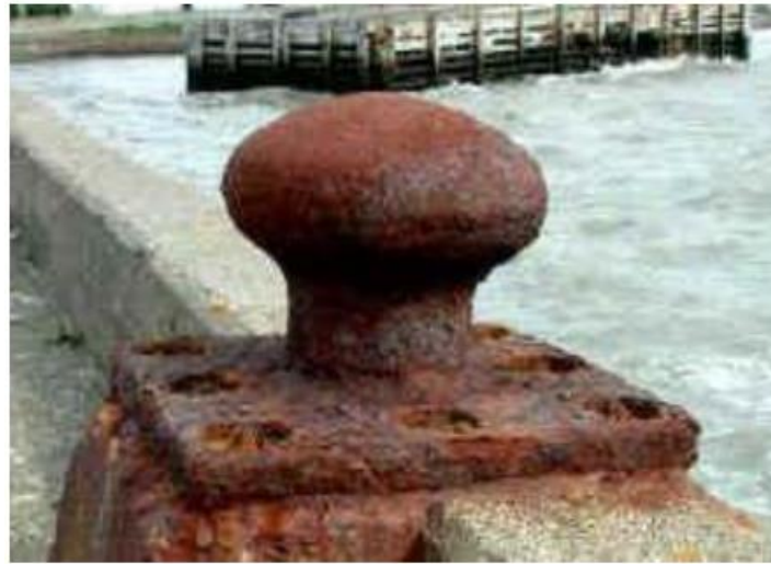
Figure 2.8 Uniform corrosion that occurs (Lazzari, 2017)
