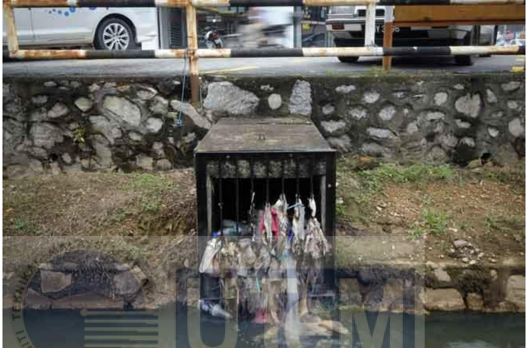
Figure 3 Example of trash clogging.
