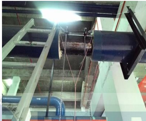
Figure 3.9: Flow meter clamp on chilled water pipe header
