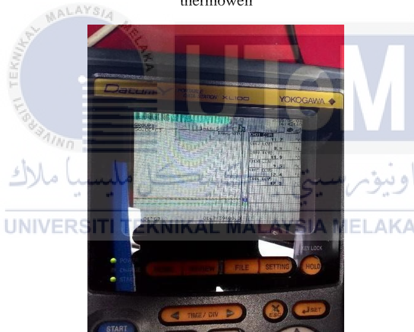
Figure 3.12: Data logger showing Air-Cooled Chiller of chilled water supply and return temperature
