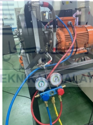
Figure 3.4 Manifold Gauge to Measured Amount of Refrigerant
