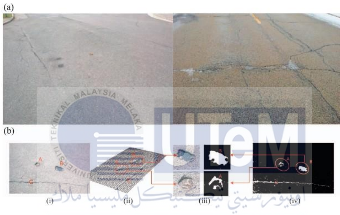
Figure 8 (a) Sample wide area 2D-image frames acquired using smartphone. (b) Selected image tile visualization and detection of potholes and linear distresses on asphalt pavements (Ouma & Hahn, 2017).
