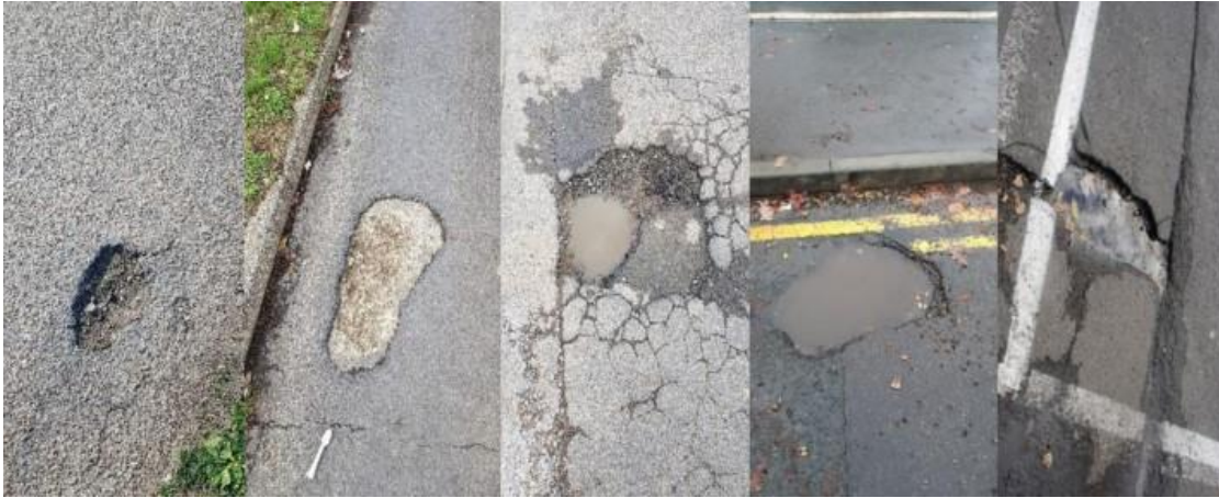
Figure 7 Different pictures of potholes (Dib et al., 2023).
