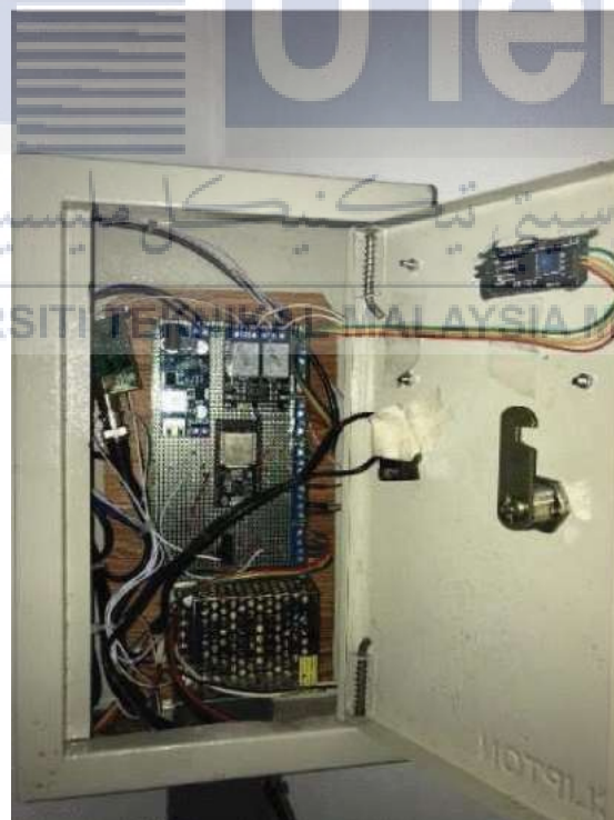
Figure 2.8: Hardware circuit inside panel box
