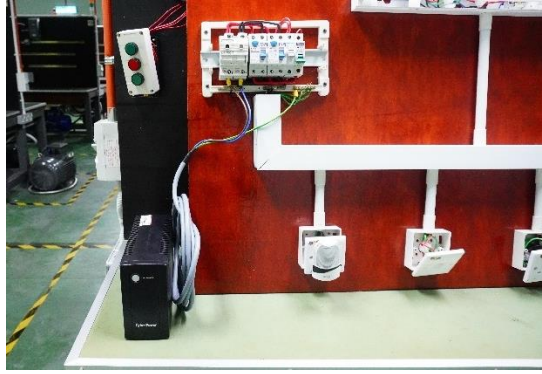
Figure 3-13 Uninterruptible Power Supply (UPS) As Main Supply
