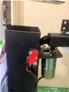
Figure 3.11 Limit switch for motor 1
