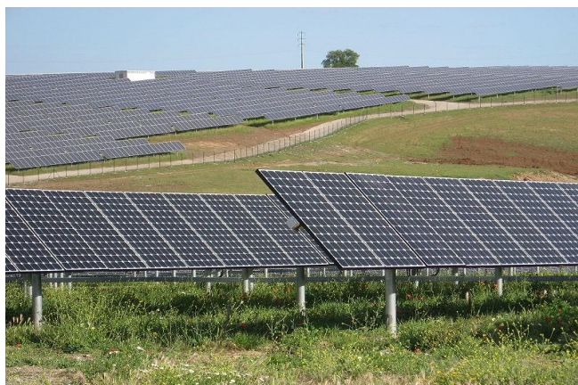
Figure 2.4 – Solar panel in big scale.
