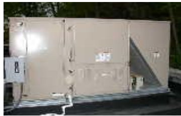
Rajah 2.2: AHU room
