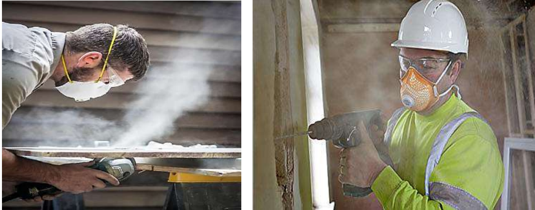
Figure 1.1 The employees are exposed to contaminants while working
