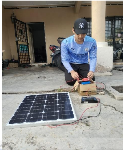
Figure 4.11: Collecting the Solar Data for Charging Phase
