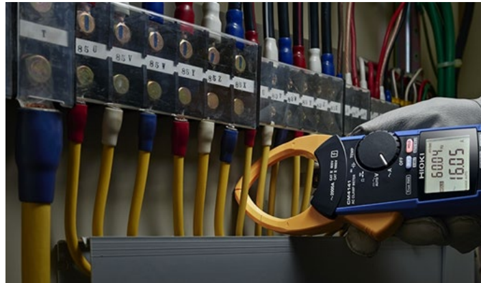
Figure 2.15 Measuring using clamp meter. (Rivers, 2022)
