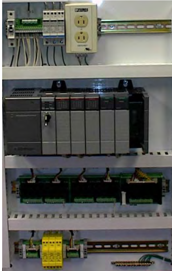
Figure 4.3.1(b): Control Panel with PLC
