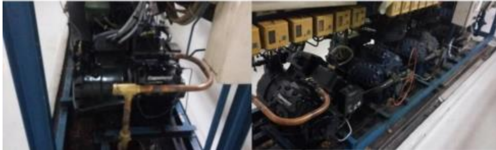
Figure 2-8 A Digital Semi Hermetic Compressor Application At Supermarket.
