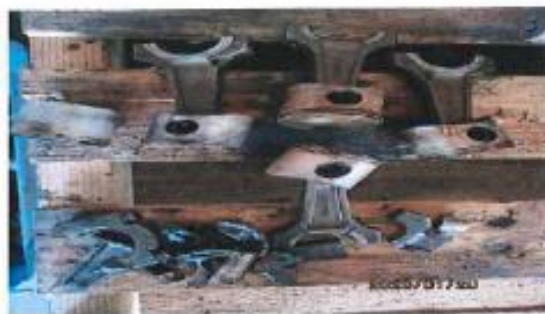
Figure 4-2 Damaged Pistons (by HVAC experts maintenance reports)
