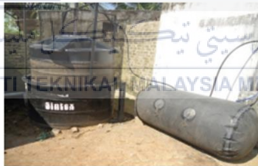
Figure 2.31: Elastic balloon Biogas storage
