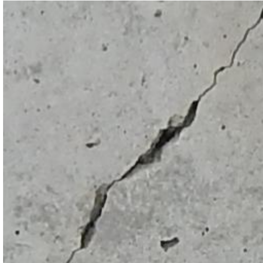
Figure 3.11: Moderate crack image.
