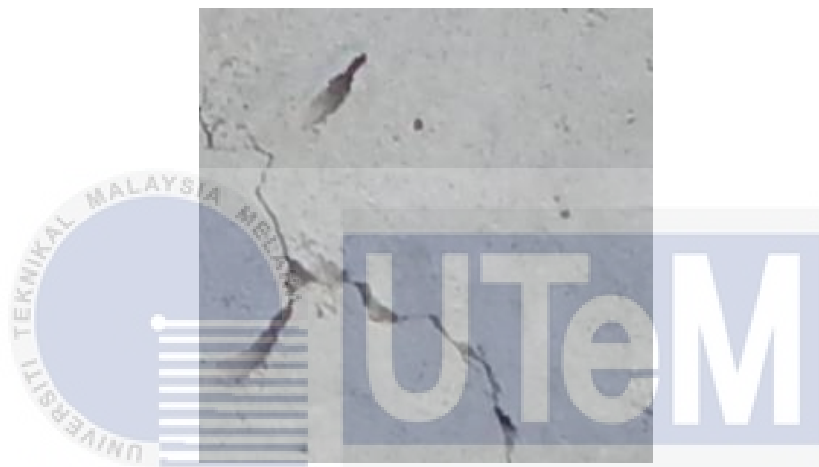
Figure 3.3: Sample images of crack concrete surface.
