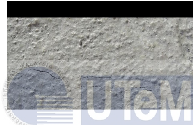
Figure 2.2: Minor crack sample from the source (Kaish et al., 2018).
