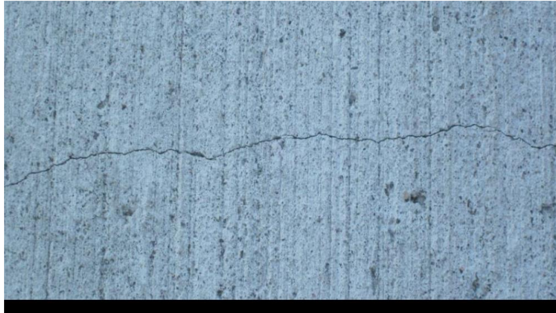
Figure 2.3: Moderate crack sample from the source (Kaish et al., 2018).
