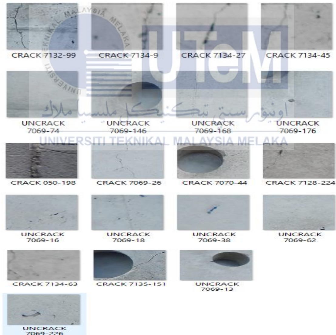
Figure 3.20: Random crack and non-crack dataset for classification test.
