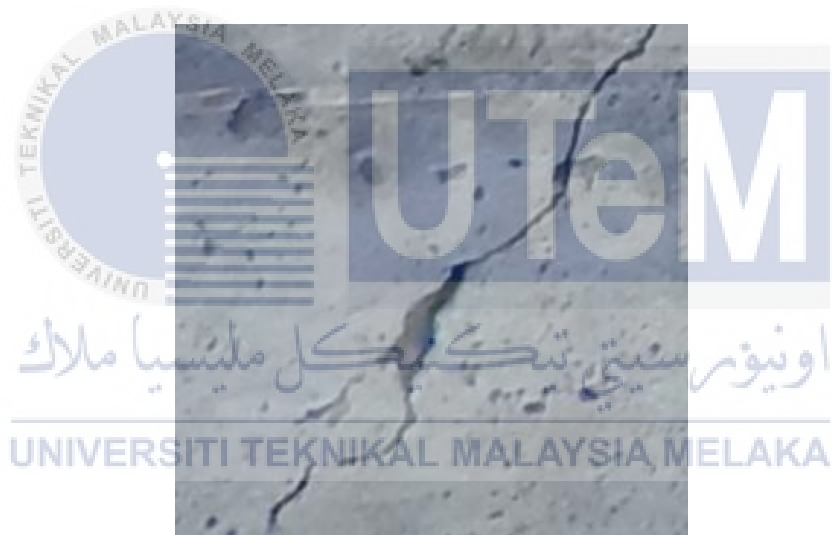
Figure 3.12: Severe crack image.
