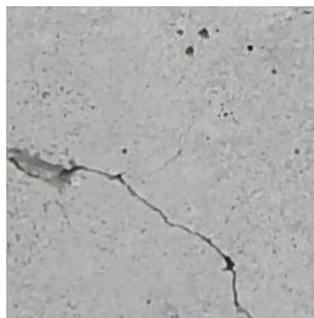
Figure 3.4: Sample images of crack concrete surface.
