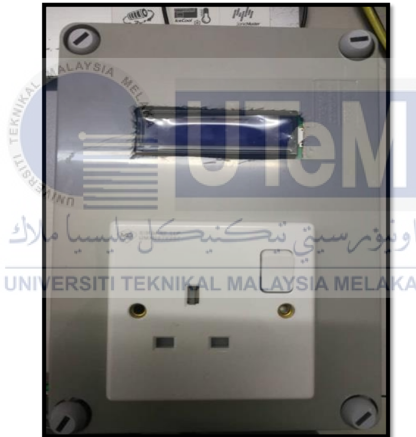
Figure 4.7: Notification Electric Usage Meter
