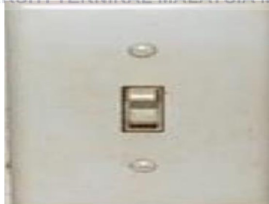
Figure 2.2 (b) 1920's switch light
