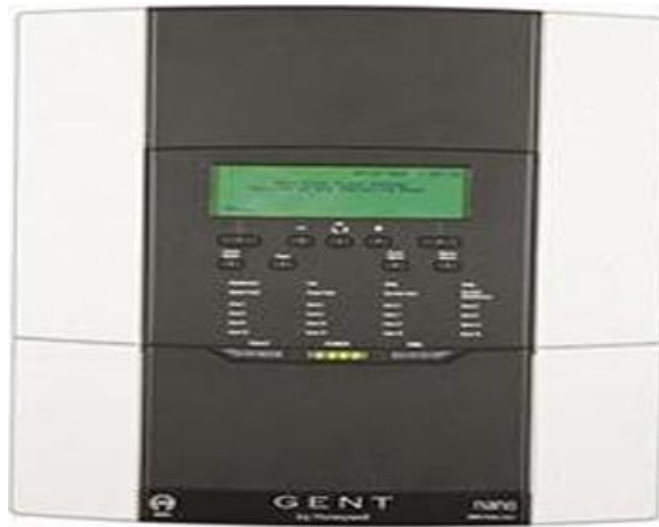
Figure 1. 4: Addressable Fire alarm control panel
