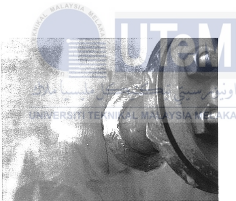
Figure 2.1(d): Cracked Vessel due to SBC
