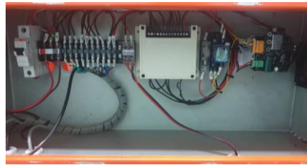
Figure 5: controller C2L unit
