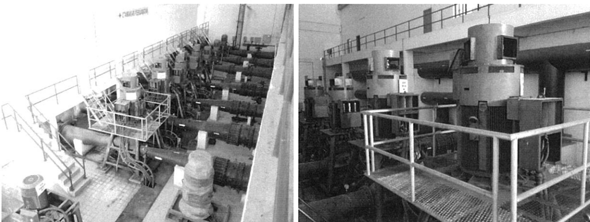
Figure 1.3.1: Centrifugal Pumps at Loji Air Bertam, SAMB
