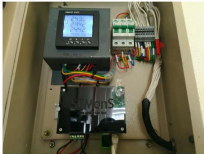
Figure 3.3: Smart Energy Meter and SEMonS wireless IoT module.
