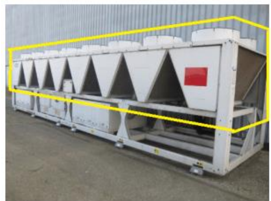
Figure 2.4(b) : Air cooled chiller condenser
