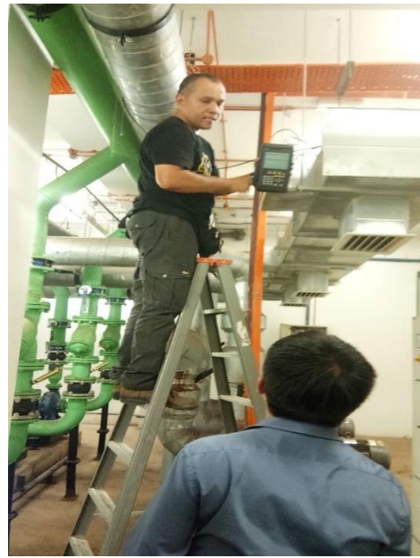
Flowrate was measured using ultrasonic flow meter
