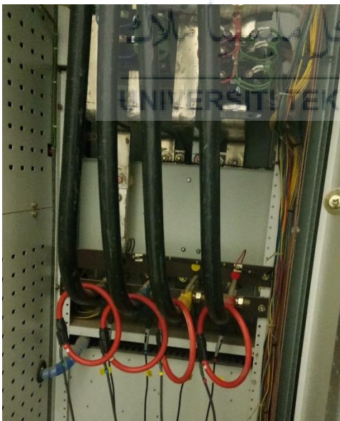
Various power of the chiller was clamped
